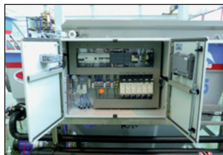
Electrical and pneumatic control in the same cabinet.
